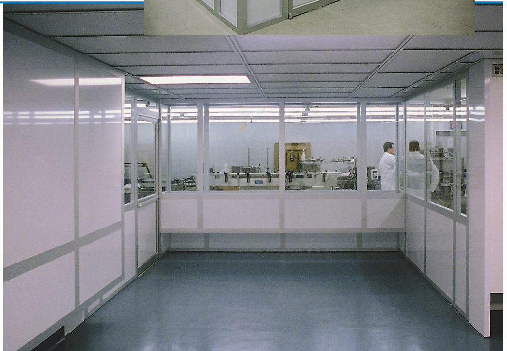
Exterior (top) and Interior (bottom) view of Lasco Services Biologic Cleanroom with elevated return air chases.
